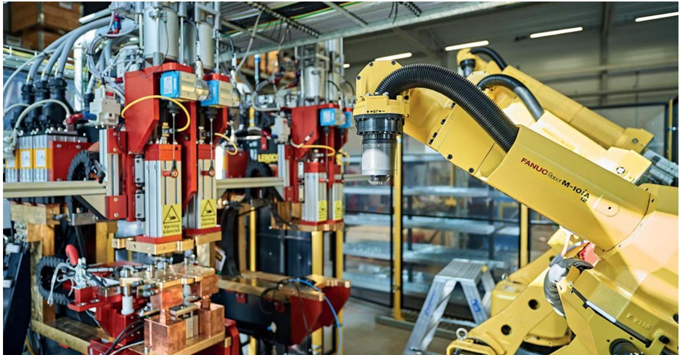
Nut welding cell during development. To the left, Lerocon's equipment for resistance welding; to the right, two TC20-IDs
